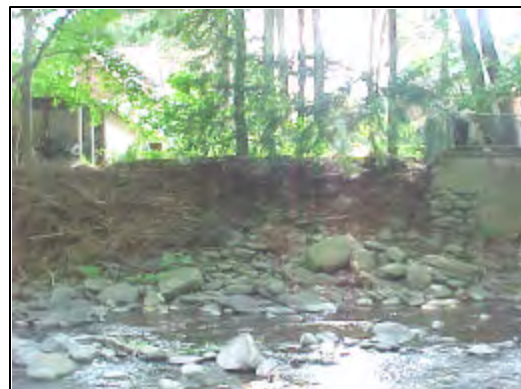
Figure 19 Erosion on right stream bank
