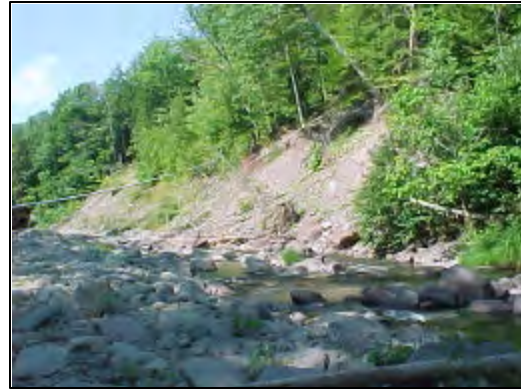
Figure 12 Bank erosion site #25
