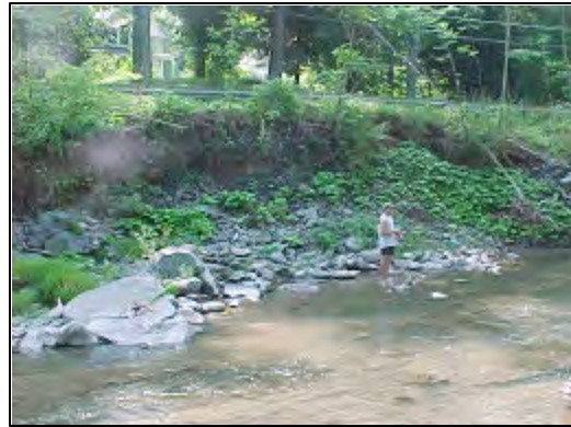
Figure 14 Bank erosion site #26
