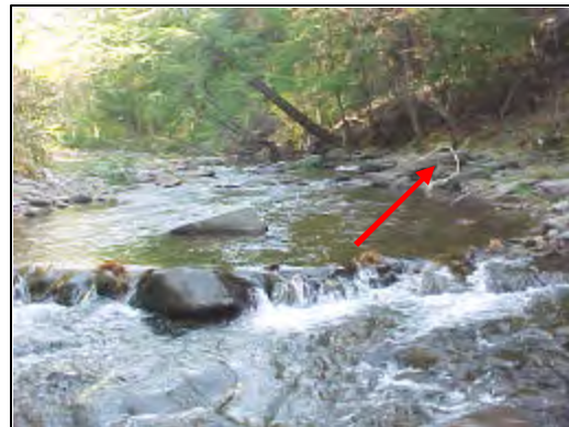
Figure 9 Cross-section 156, minor toe erosion Stream Type F3 Looking Upstream
