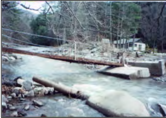
Figure 4 Bridge At Weiss Road April 24, 2000
