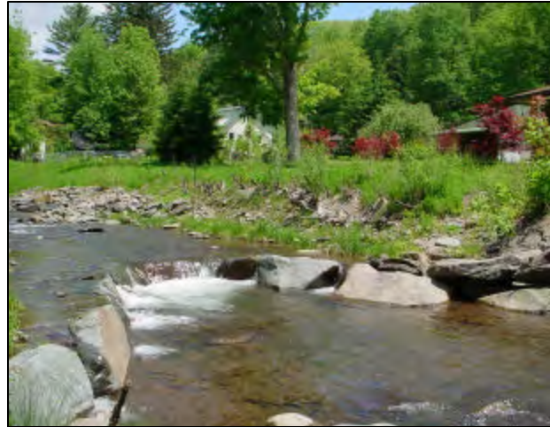
Figure 19 A cross vane at the stream restoration site on Broadstreet Hollow. Notice how the cross vane redirects stream flow into the center of the channel, away from the banks.
