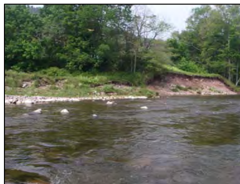
Left bank downstream of Deming Road Bridge – site for bank stabilization and buffer planting with shrubs and trees.
