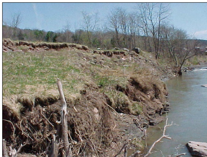
Image of downstream bank erosion and failure.
