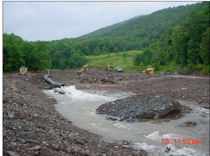
Phase I dewatering outlet.
