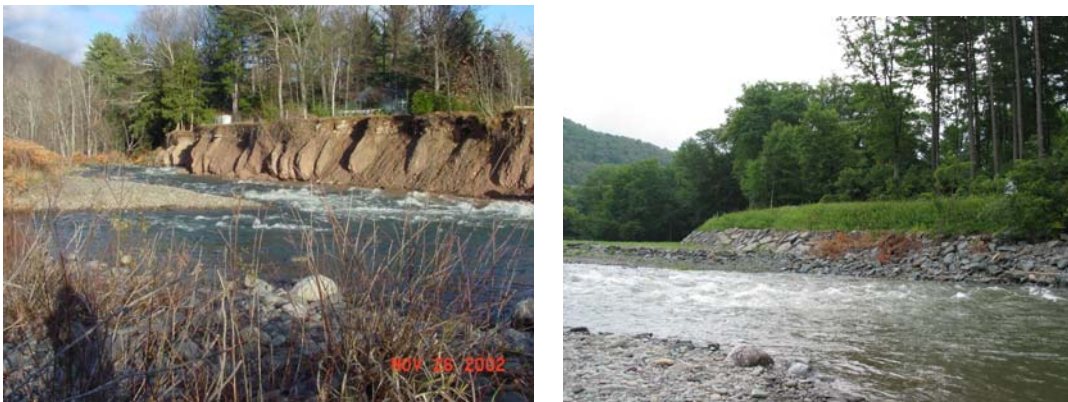
Erosion in the Esopus Creek (left) and the same bank post-restoration with bank armor including a vegetation component (Vegetated Reinforced Slope Stabilization) (right). This project also included in-stream structures that aren't shown in these photos.
