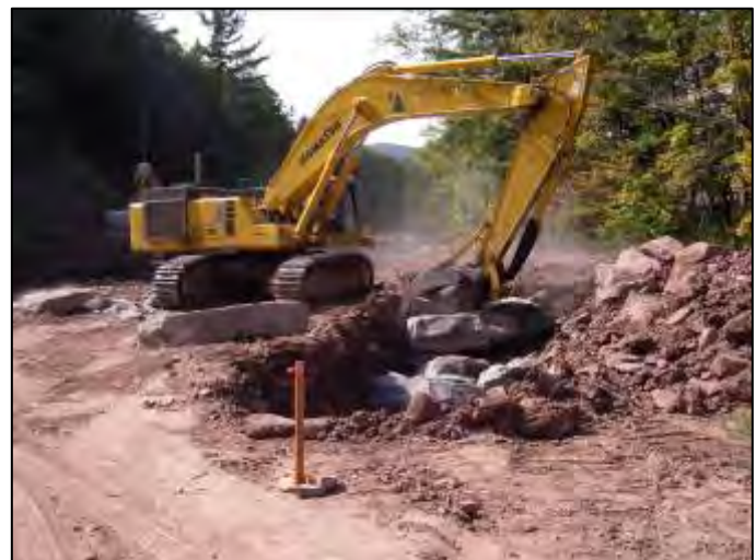
Excavation and construction of a cross vane arm near the center of project reach.
