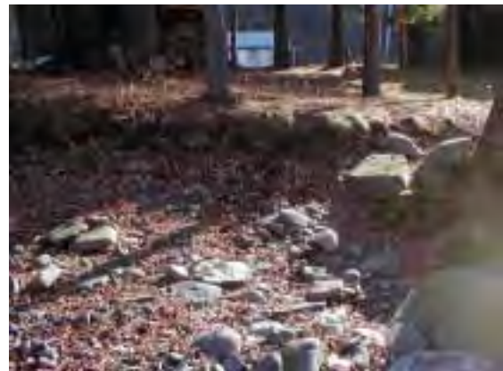
Photo 12. Low eroding left bank, just downstream from Timberlake Road bridge near the top of MU4, stream flow is from left to right.
