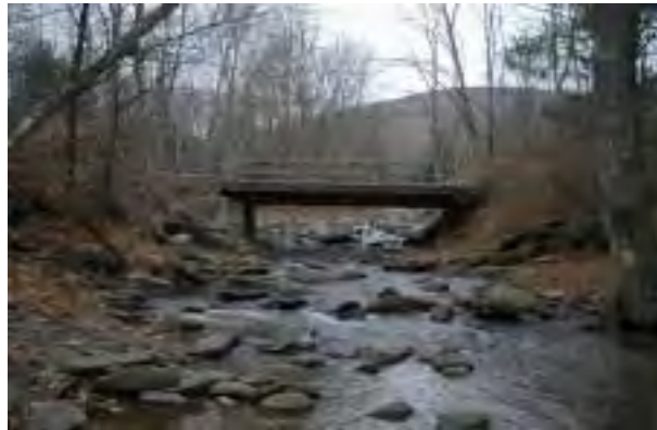
Photo 4. Looking upstream into the top of MU4 at the Timberlake Road bridge, County BIN 3-20124-0.
