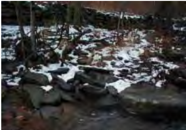
Photo 7. Old mill race and dam wall, right bank upstream of County bridge 3-20122-0. Flow is from right to left.
