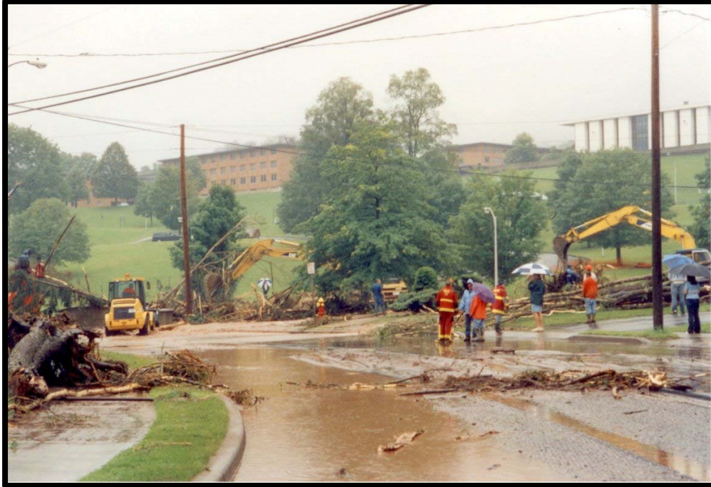
Figure 28: Photo of Flooding Aftermath. Looking West at Main Street Bridge
